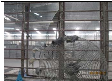
(19) Broken glass window in moulding workshop
